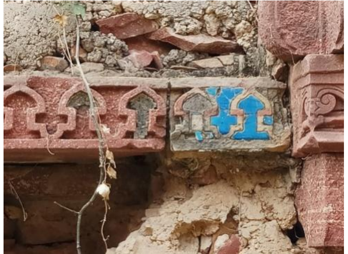
Surviving band of blue glazed work
